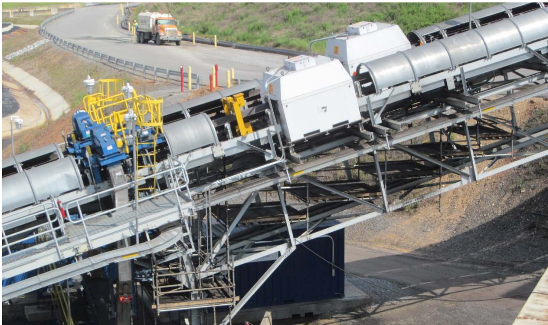
Model 730 FSEAs at Duke Energy - Cliffside Steam Station, Rutherford County, North Carolina
